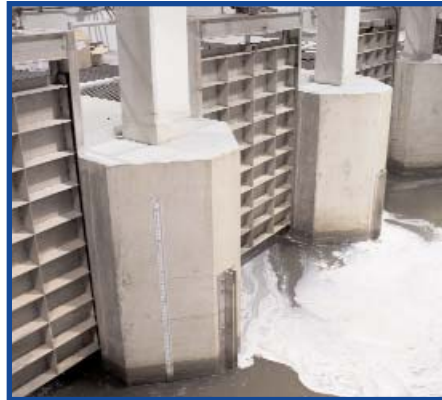
Influent (raw sewage) following the screening process. From here the wastewater goes through the main pumps to the settling tanks for primary treatment.
