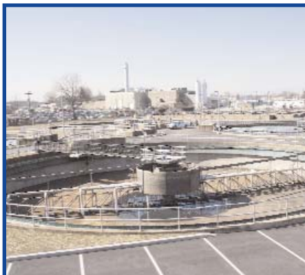
Final Clarifier (settling tank). This is considered "secondary treatment." Four clarifiers were rebuilt as part of the upgrade and two new ones were added.
