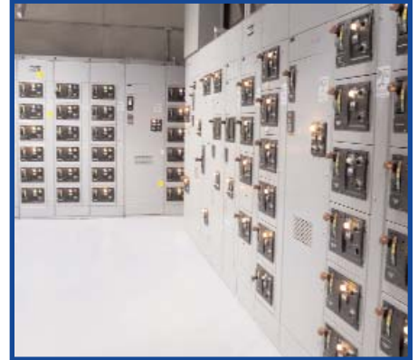
A Motor Control Center (MCC) in the Co-Generation/ Sludge Drying Facility.
