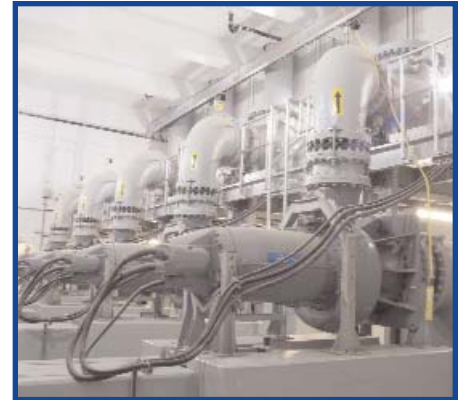
Main influent sewage pumps. Each pump can process 27MGD. Four are in "operations" mode and one is a standby pump.
