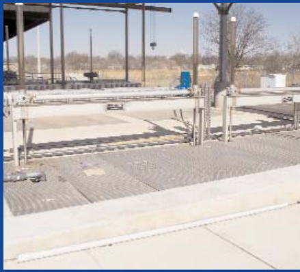
Ultraviolet Disinfection Facilities. UV lamps are underground; final effluent is exposed to UV light to essentially disrupt the DNA of any remaining bacteria.
