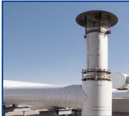
Exhaust stacks from the gensets at the Co-Gen Facility. Each stack incorporates a “silencer,” which essentially acts like a muffler.
