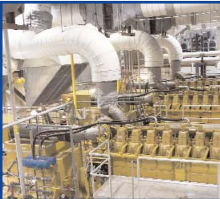
The Co-gen facility has four “Caterpillar gensets.” Each is capable of producing 1.55 megawatts (MW) for a total of 6.2MW of potential power.
