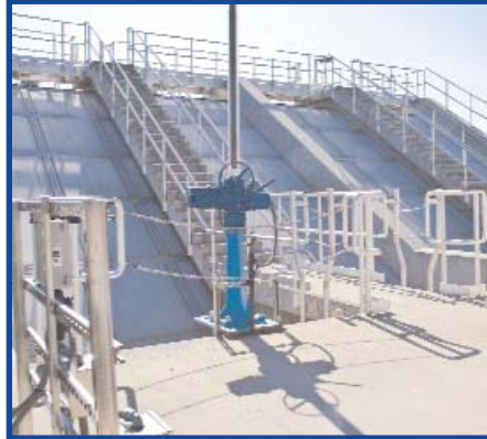
Effluent Screw pumps. There are four — each capable of pumping 35MGD. The final effluent flows to the Arthur Kill on its own; pumps are only activated during heavy rain or high tide.
