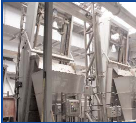
Fine Screens at the Headworks facility. These are used to remove smaller debris — following Coarse Screens — from the wastewater before primary treatment.
