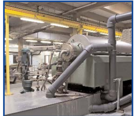
Dewatering centrifuges prior to the sludge drying facility. The centrifuges spin the sludge to mechanically remove as much water as possible.
