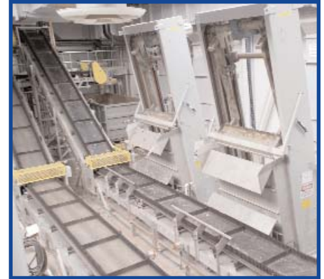
Coarse Screens at the Headworks facility. These are used to remove larger debris from the wastewater before primary treatment.
