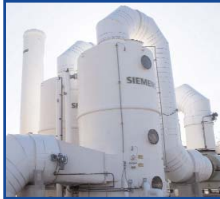
Odor Control System (OCS) at the Headworks facility (where preliminary treatment takes place). The OCS conditions the exhaust air leaving the facility.
